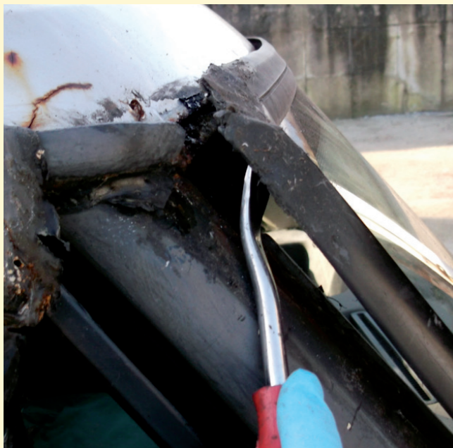
No adhesion between windscreen and aperture and severe damage caused by corrosion
